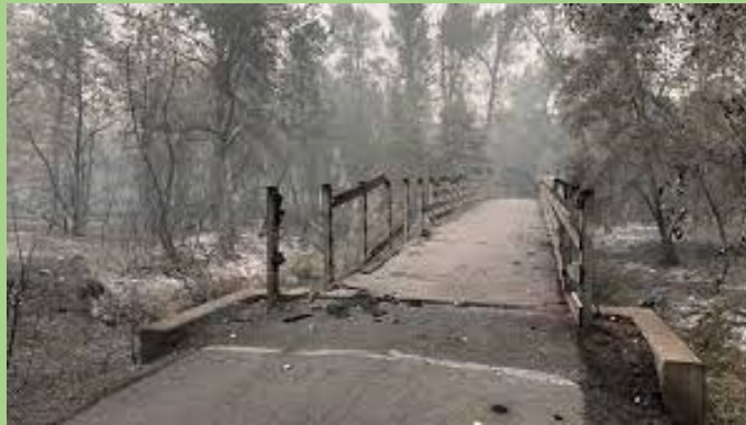
Figure 3. Burned bridge along the Bear Creek Greenway from the Almeda Fire. Image source: Jackson County Emergency Management
